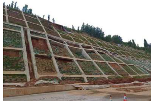
(b) Lixi highway landslide
