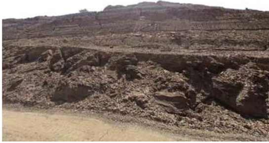
(a) Jinyang highway landslide
